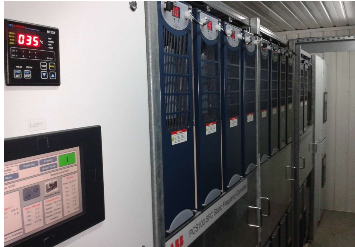
Shore-to-ship power converters
