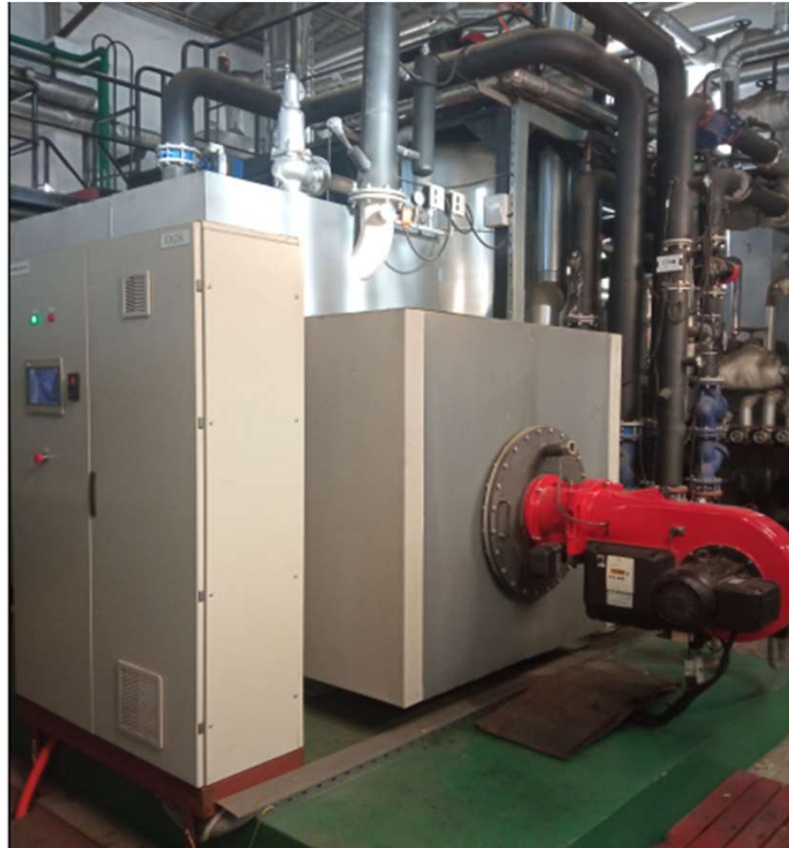
Central boiler room – Water heater boiler
