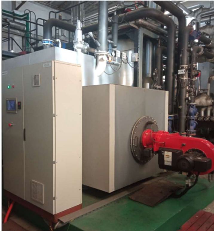
Central boiler room – Water heater boiler
