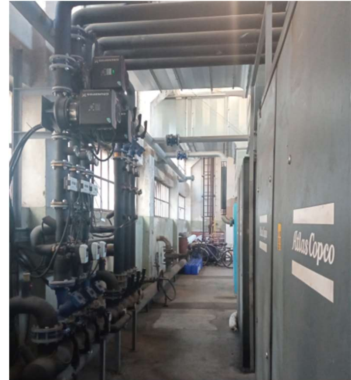
Waste heat from compressor
